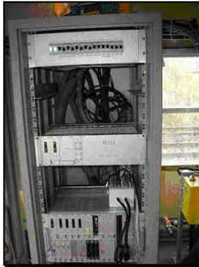
Fig.3 : The main cabinet
